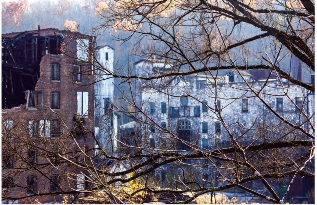
Old Crow Distillery buildings, Woodford County. From the road in autumn one can see the main distillery in the center, the grain elevator building to the left, and the remains of one of the warehouses in the left foreground.
